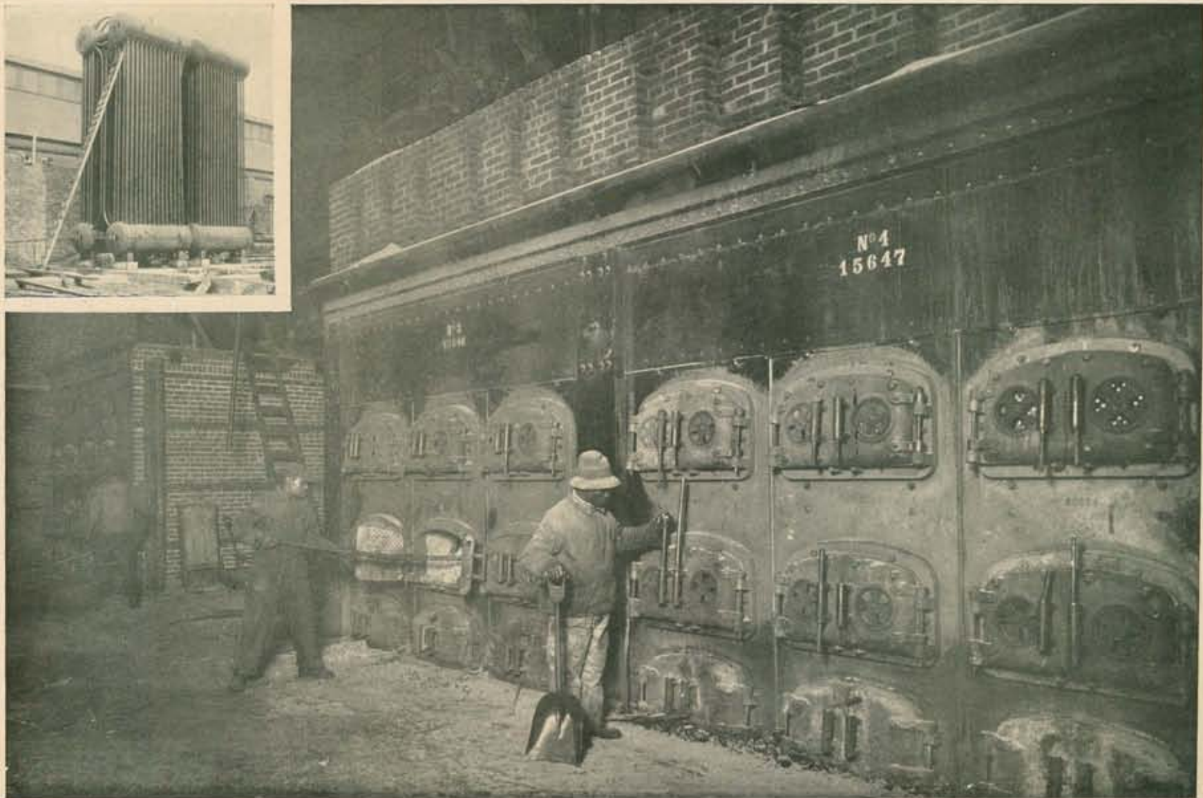
"BABCOCK & WILCOX"—WATER TUBE BOILERS ( Rust-type ) THREE WITH "DUTCH-OVENS"—CONVEYOR FEED.
